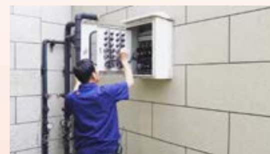
◆ Hardware equipment maintenance at communities
