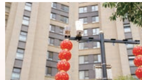
◆ Monitoring the hidden hazards of the facades
