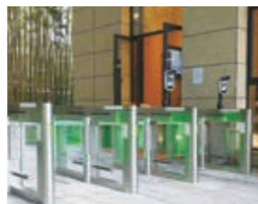
◆ Smart access control system
