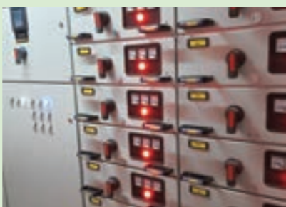
◆ Smart Ammeter Reading System
